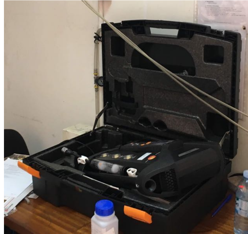
Incorrect CO 2 analyzer (0-25% +/- 0.5%)
